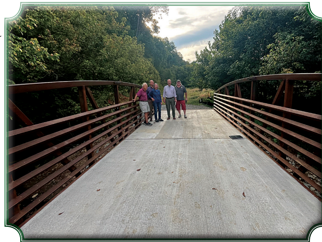
From left to right: Project leader Herb Shulhafer, Prospect CAO John Carter, Parks Committee leader Linda Wardell, Mayor Doug Farnsley and Public Works Director Ron Cundiff look over the nearly completed pedestrian bridge in Hunting Creek Park.
